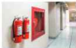
FIRE FIGHTING EQUIPMENTS
